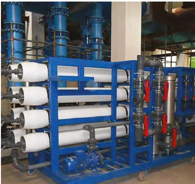
Reverse Osmosis Plant (for potable water)
