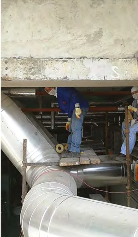
Exhaust Pipe Ducting + Cladding
