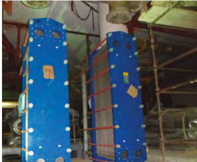
Hot Water Heat Exchangers
