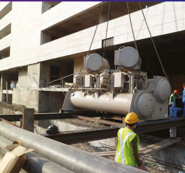
Unloading the DAIKIN Electric Chillers
